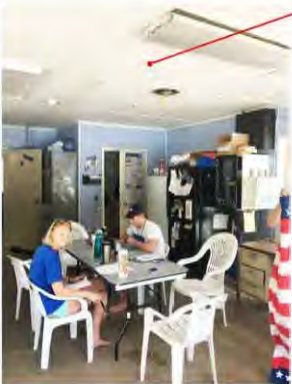
Staff area is inadequate poorly lit, does not offer space for adequate storage, staff meetings, private area for staff breaks, access to staff area does not meet accessibility code requirements
