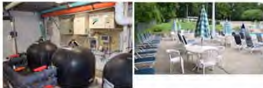
Other renovations include site lighting, public address system, diving equipment, terraces, rest areas, and upgrades to the chlorination and plumbing systems.
