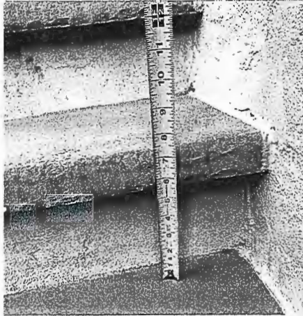
Figure 2: Front Porch Stairs within Construction Code Distance ( \leq 8 \frac{1}{4} inches)
