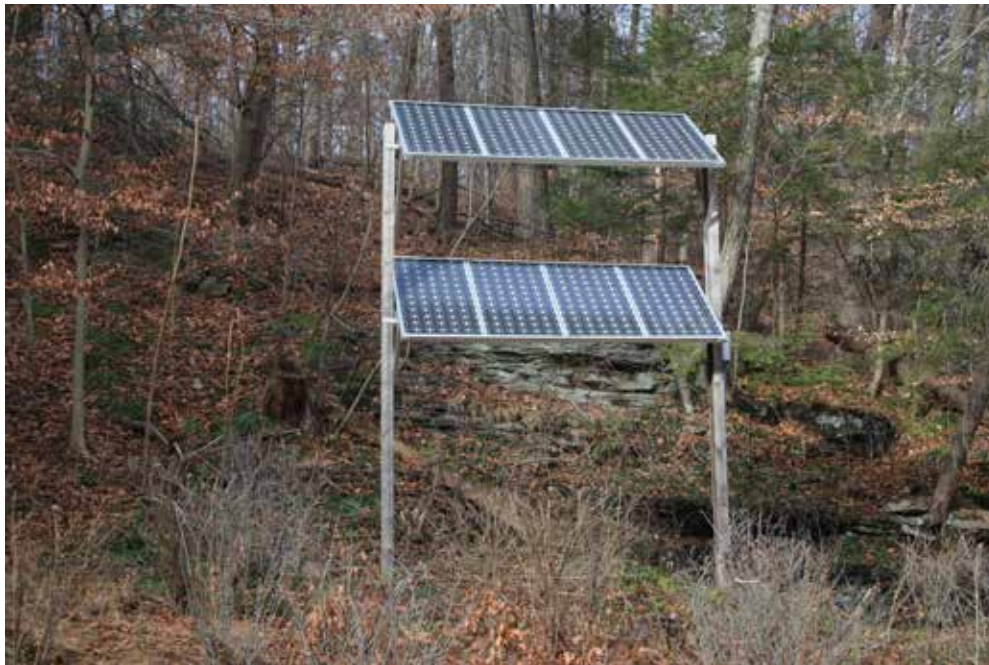
Solar Energy System, Ground-Mounted
