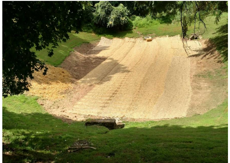
Stormwater improvements such as the reestablishment of a basin grade are performed by the Engineering Department's Construction Services Team
