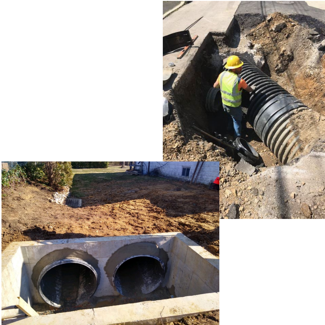
Figure 2-8: Hamel and Monroe Flood Mitigation Project increasing drainage system capacity and pipe longevity
