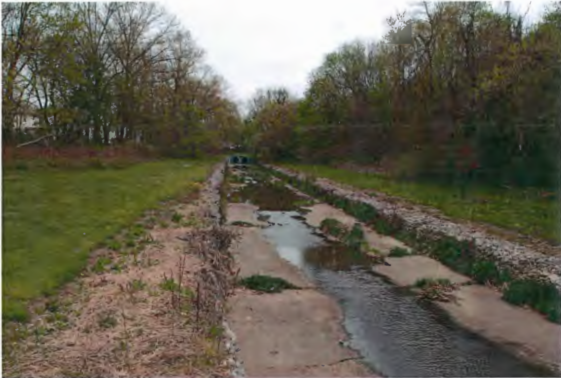
Figure 3: Concrete and gabion lining of Sandy Run Creek in Grove Park, Abington Township
