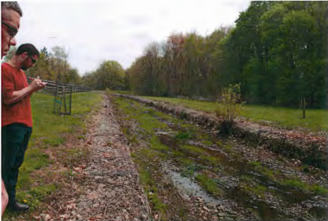
Figure 4: Gabion lined Sandy Run Creek downstream of concrete lined segment in Grove Park, Abington Township
