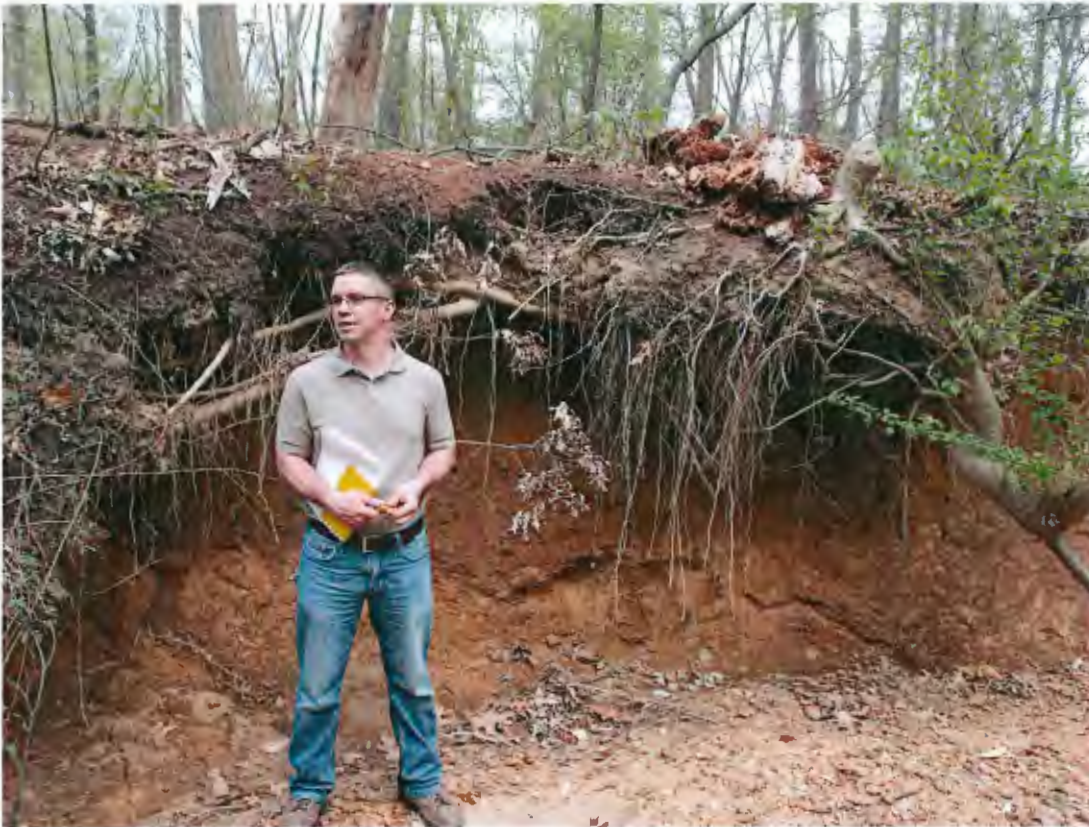
Figure 8: Severely eroded and undercut bank in an intermittent stream in Ardsley Wildlife Sanctuary, Abington Township
