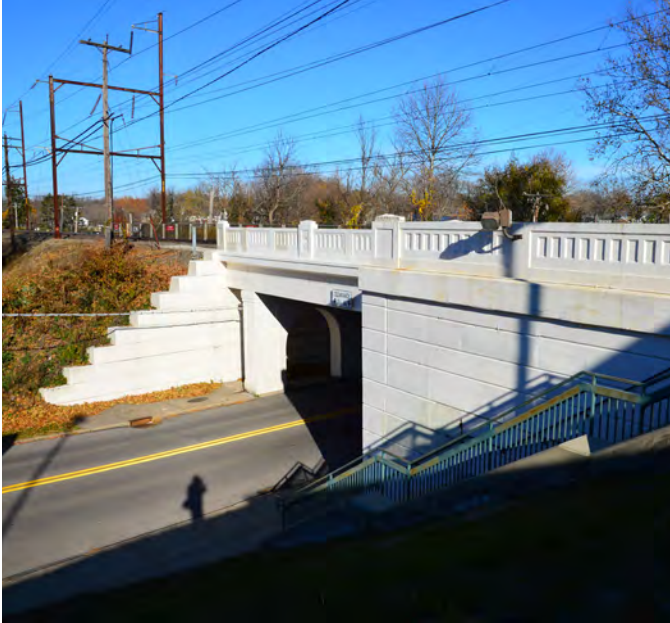
Rail bridge and Stairs to North Hills Station (inbound side) from N. Hills Ave
